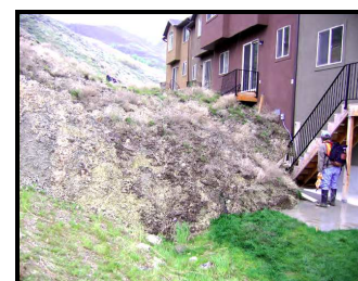
Townhouse damaged by a landslide in Cedar Hills, northern Utah County, April 28, 2005.
